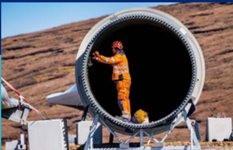
Final preparations are made to one of the turbine blades at Viking wind farm
