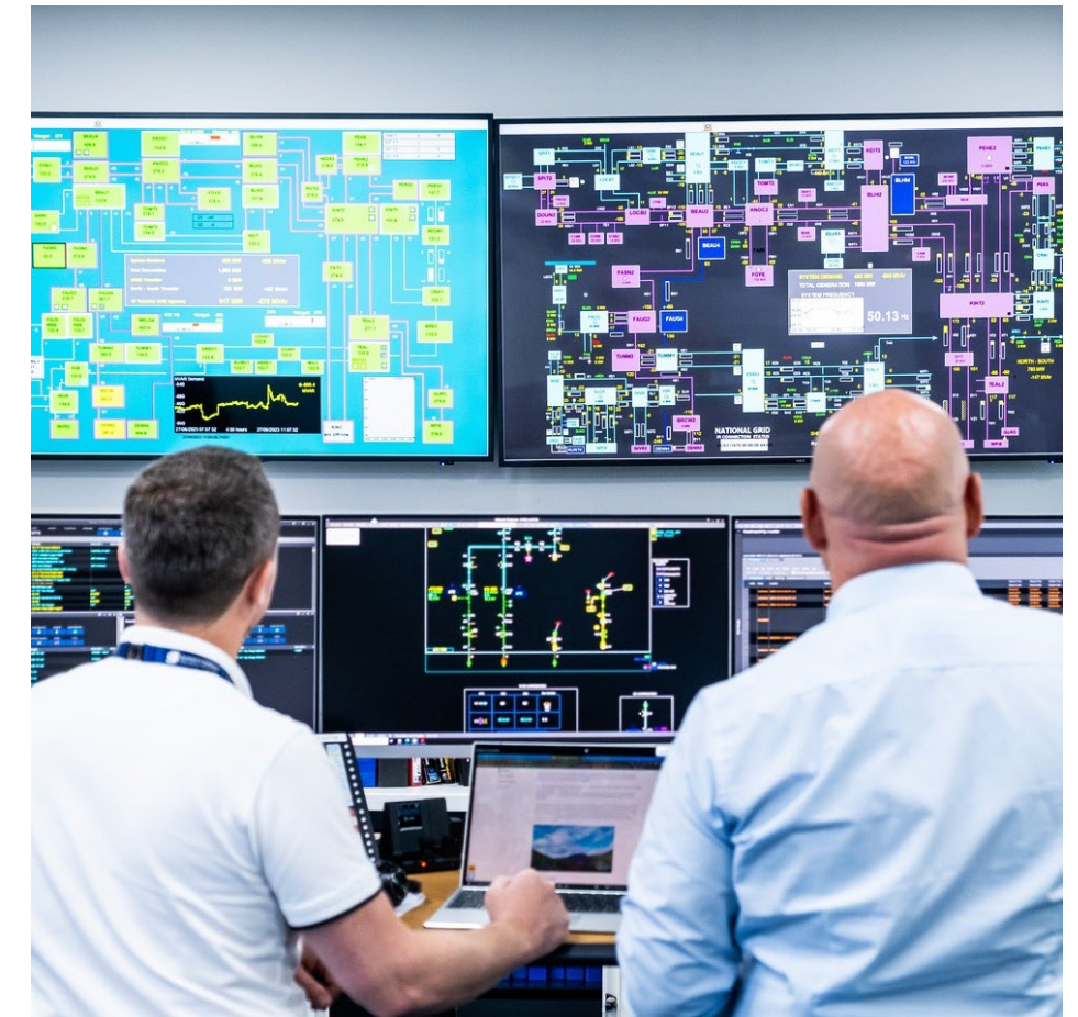
SSEN Transmission control room
