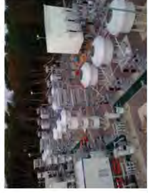
Example AC Substation
