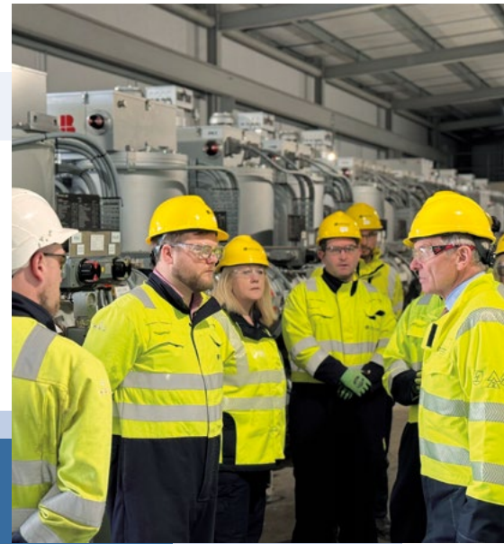
Members of the Board during their visit to the Iver primary substation
